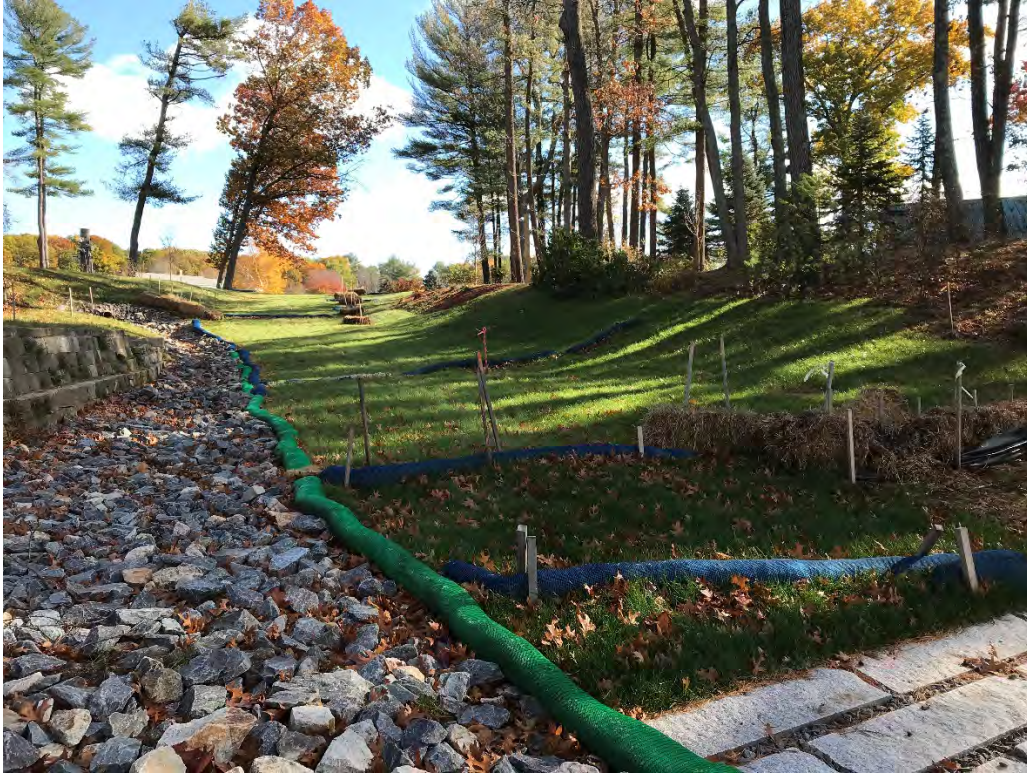
Fig 3: Slope above the manhole at Gundalow Landing/east side of the bay. Viewing east. (11-03-20)
