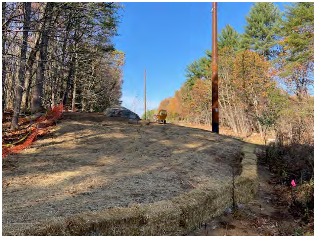
Fig 8: Access route between Str. 89 and wetland DW22 graded and mulched with straw. Viewing northwest. (11-04-20)
